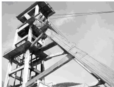
Fig.1. . Installation tower „ Auxiliary well no. 2 “
